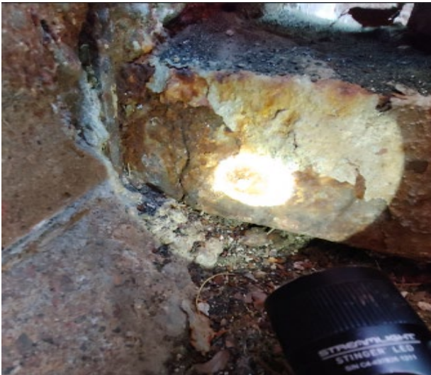
Figure 3. Crack in bottom plate at Lock 4
