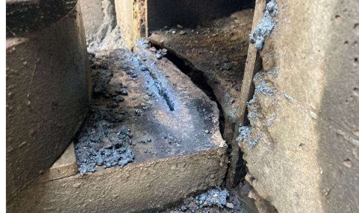
Figure 2. Fractured Bottom Plate at Lock 5A
